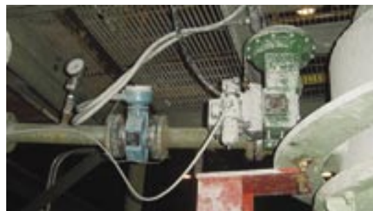
Wash water feed line into the ReCyclone, complete with control valve, flow meter and pressure gauge.
